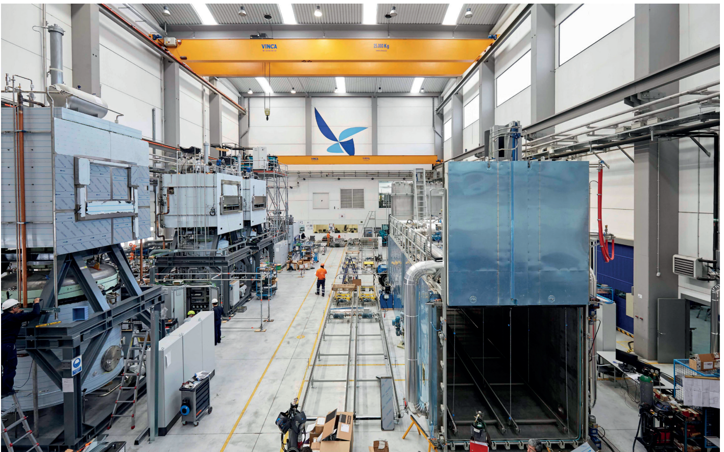
Sterilization equipment at Telstar's facility in Terrassa
